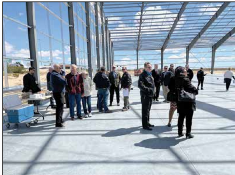
Visitors inspect the steel superstructure of future home of the Flight Test Museum that is under construction outside the West Gate at Edwards Air Force Base Calif.
