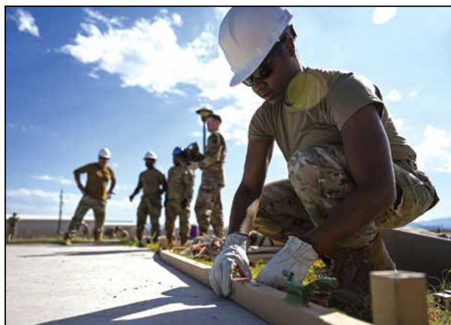
A U.S. Airman assigned to the 355th Civil Engineer Squadron, assembles the structure of an Alaska Small Shelter System at Davis-Monthan Air Force Base, Arizona, Aug. 30, 2023. Airmen were split into teams of 12 with one person from each CE career field to build the shelters during a CE Readiness Challenge.
