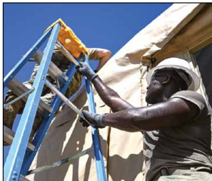
U.S. Airmen assigned to the 355th Civil Engineer Squadron, finish assembling a hardened door to an Alaska Small Shelter System at Davis-Monthan Air Force Base, Arizona, Aug. 30, 2023. Airmen collaborated with other CE career fields during a CE Readiness Challenge.
