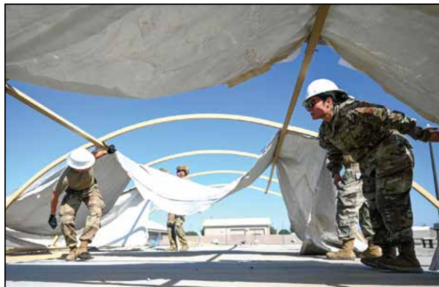
U.S. Airmen assigned to the 355th Civil Engineer Squadron assemble an Alaska Small Shelter System at Davis-Monthan Air Force Base, Arizona, Aug. 30, 2023. Airmen assembled the shelters as the first event of a CE Readiness Challenge.
